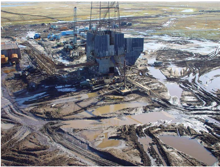
Figure 6. Test well drilling in the Varandey area. Large tundra spots are degraded through such activities. Photo: Yasavey, September 2002.
